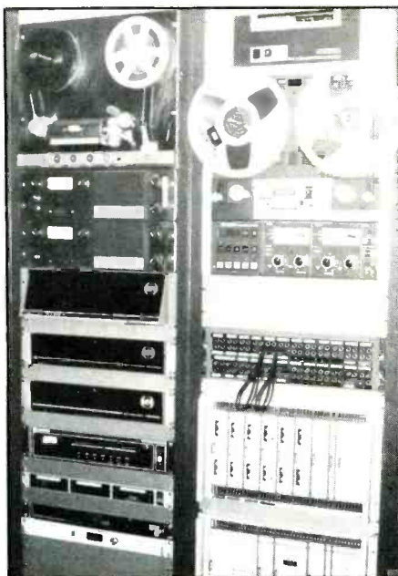
Satellite receiver installation. Left rack from bottom: Bottom two items used to pick up music for transmission on SCA. Next two panels receive CNN video and audio. Next three items used with UPI. Right rack from bottom: First item is receiver typical of ABC, CBS, NBC & RKO. Next items are the decoders for audio/data. Each strip has two channels. Jack field connects receiver to other parts at station. Tape recorders used for taping from satellites. (Courtesy of WBAL, Manucy photo)
